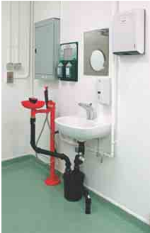
Emergency eye wash
